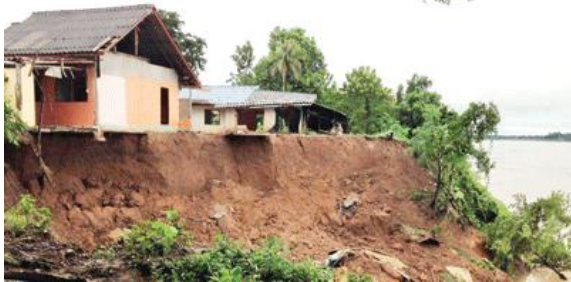
Five houses were demolished when this riverbank collapsed in Thaphabath district, Borikhamxay province, on Sunday. -- Photo Pathedlao Lao Facebook
